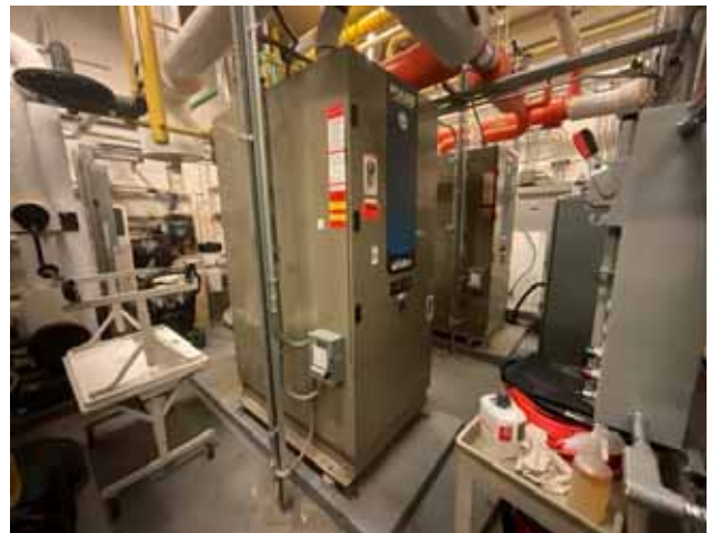
22 - HVAC HEATING BOILERS
