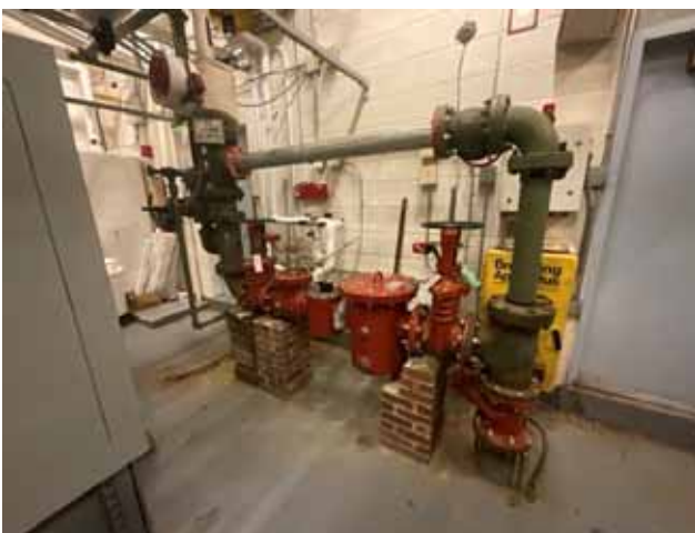
29 - FIRE BACKFLOW PREVENTER
