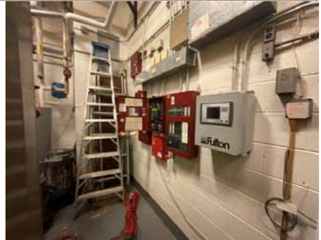
32 - FIRE ALARM CONTROL PANEL
