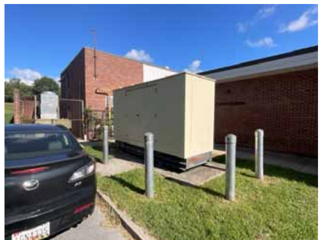
30 - EMERGENCY POWER GENERATOR
