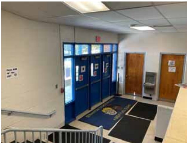
33 - FIRE ALARM SYSTEM DEVICES
